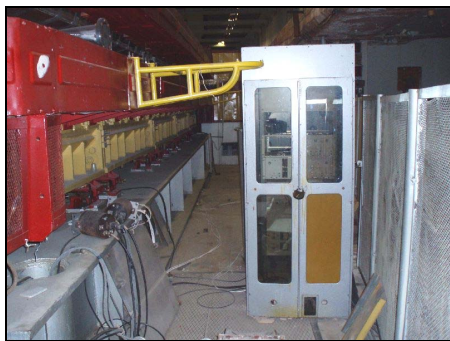
Figure 12: Shelf with a low-level electronics near SS #2 in ring hall of the U70.
