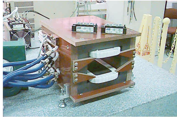
Fig. 1 Picture of the magnet with the IGBTs on top.
