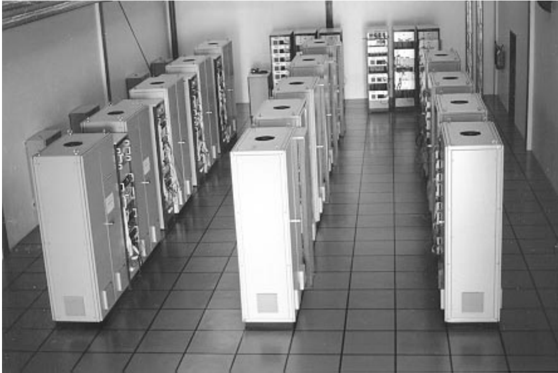
Figure 1: power supply room
