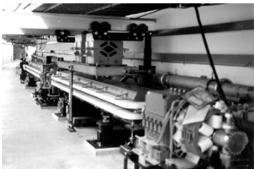
Figure 3 Installation of the first HER arc cell with operating Cu vacuum chamber. A prototype LER raft is mounted above.
