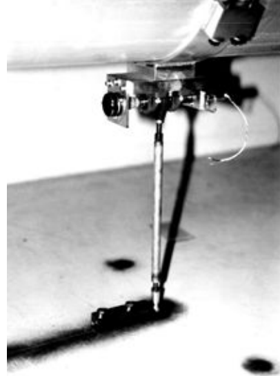
Figure 3: Close-up photograph of the remotely control motorized CAM to move the accelerating structure center by +/- 1 mm. Both vertical and horizontal movers have been placed on 8 adjacent RF girders covering 100m of the SLAC linac.
