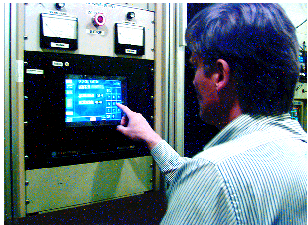
Figure 6. Programmable Logic Controller operational center for the RHEPP-II system
