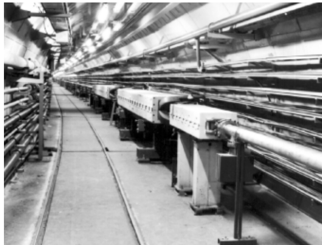
Figure 4: Beam transfer line tunnel.
