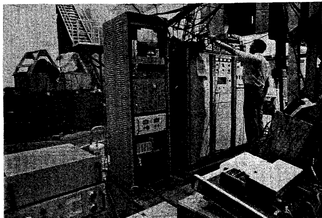
FIG. 6 -- Power supplies and auxiliary equipment for the neutron therapy cyclotron. The rf transmitter occupies three racks in front of the operator. The magnet power supply is in the rack on the left (light colored panel slightly below midpoint of the rack). Ion source power supply is on table at the lower left.
