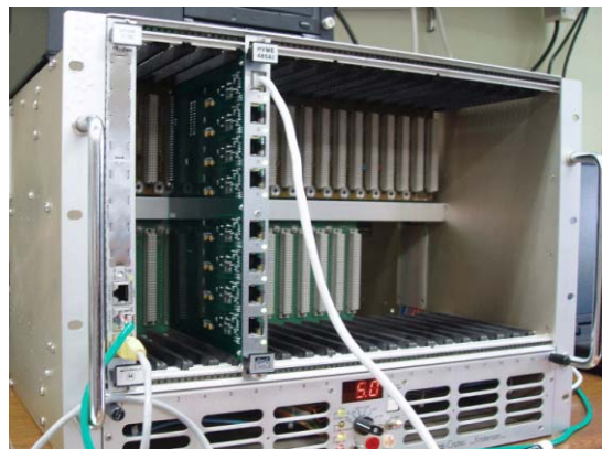
Figure 3: Picture of the VME IOC for the power supplies
