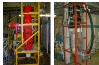
Figure 4: Existing klystron TH2104A (left) and high power water load in test stand (right).
