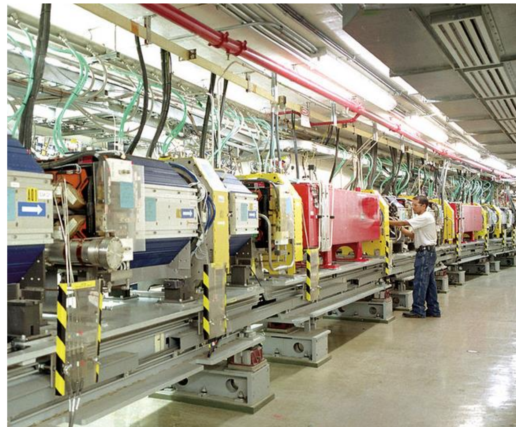
Figure 2: Photo of the APS storage ring within the accelerator enclosure [6]. Prominent in this image are the flexible tubing (aqua) serving individual accelerator components, connected to the water manifold at the ceiling. The fire sprinkler piping (painted red) is also visible along the ceiling. [Adapted under CC BY-NC-SA 2.0 license from Ref. [6].]
