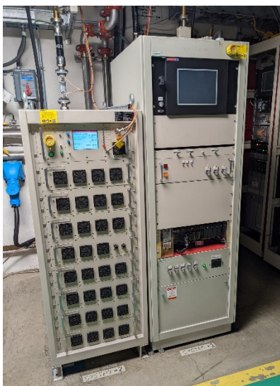
Figure 3: PAR harmonic rf amplifiers: new 10-kW SSA is shown on the left and 3-kW tube amplifier is on the right.
