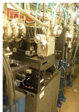
Figure 1: Installed GRID-XBPM at 27-ID FE (Looking upstream) [2].
