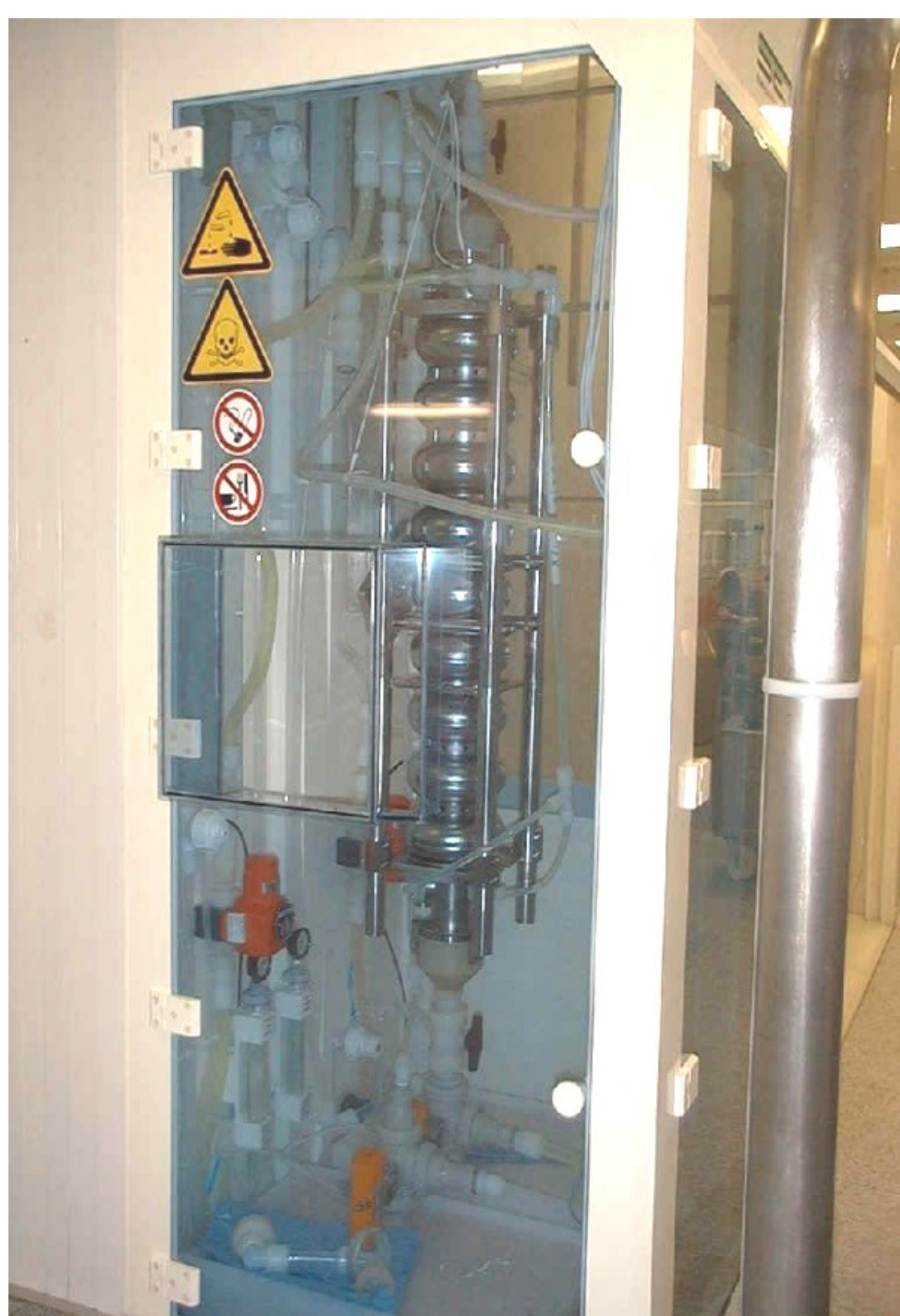
Buffered chemical polishing cabinet with an undressed nine-cell European XFEL cavity installed
