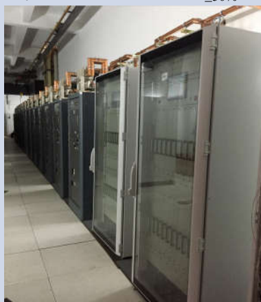
Figure 1: 325 MHz/10 kW SSA
