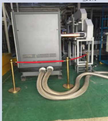
Figure 3: 650 MHz/150 kW SSA
