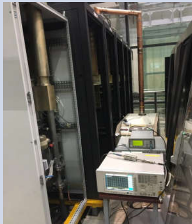
Figure 2: 325 MHz/25 kW SSA
