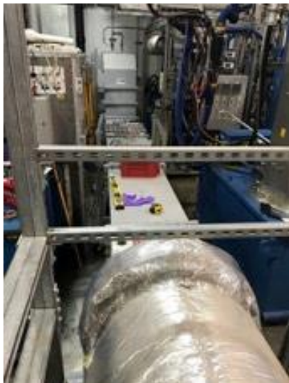
Figure 3: Test setup for the SNS warm linac high power RF.
