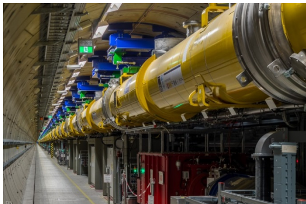
Figure 2: View into the linac tunnel with the accelerator modules suspended from the ceiling and the RF infrastructure placed below, on the floor.
