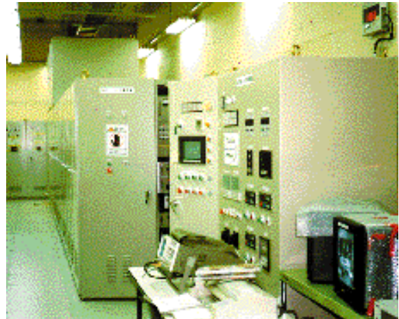
Fig. 2 The modulator installed in the electron beam sterilization facility.
