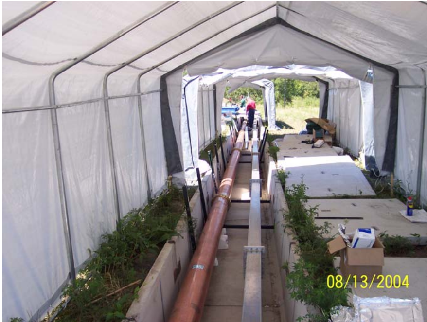
Figure 8. Picture of the installation of the 805 MHz waveguide and 201 MHz 0.233 m Coax hardline on top of linac berm looking away from linac towards the MTA.
