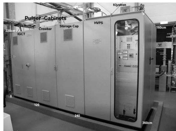
Figure 5: HVPS / Pulser cabinets of the new modulator.
