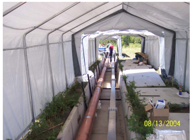
Figure 8: Picture of the high power 805 MHz and 201 MHz transmission lines at top of linac shielding being installed to the MTA.
