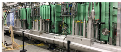
Figure 5: LS1 cryogenic transfer line (viewing the cryomodules from the side opposite that of Fig. 2).
