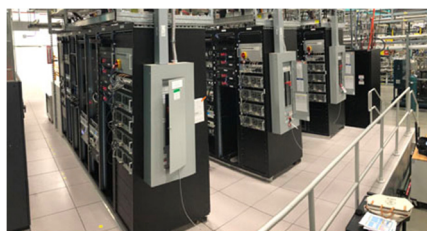
Figure 6: Racks for the \beta = 0.041 cryomodules. Each row of racks corresponds to one cryomodule.
