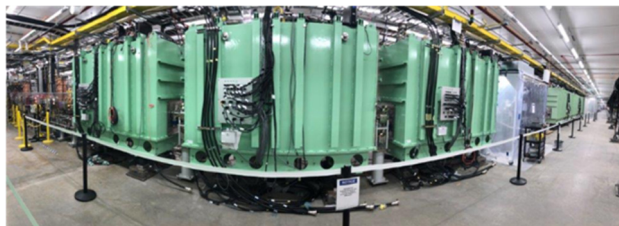
Figure 2: \beta = 0.041 cryomodules installed on beam line.
