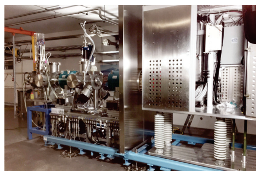
Figure 2: IS and LEBT installed in the ESS linac tunnel.
