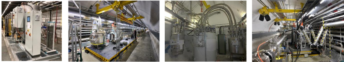
Figure 2: Surface and tunnel installation of the cryogenic, mechanical and RF infrastructure to support the crab cavity testing in the SPS-LSS6 region.
