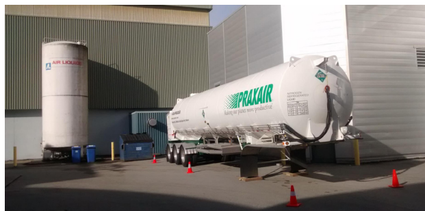
Figure 6: Trailers used for temporary LN2 storage.
