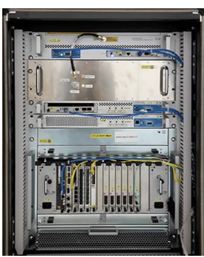
MicroTCA crate in XFEL Tunnel.
