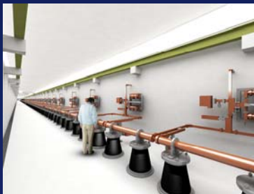
C-band accelerator consists of 128 accelerating structures
