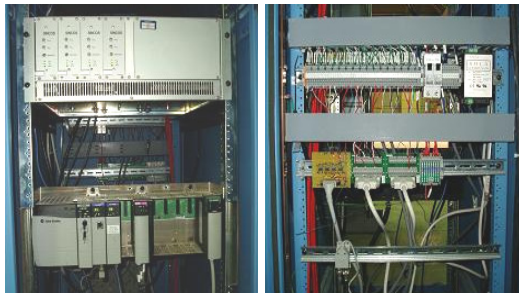
Figure 6a and 6b: Front and rear of PLC-based stepper motor control cabinet.
