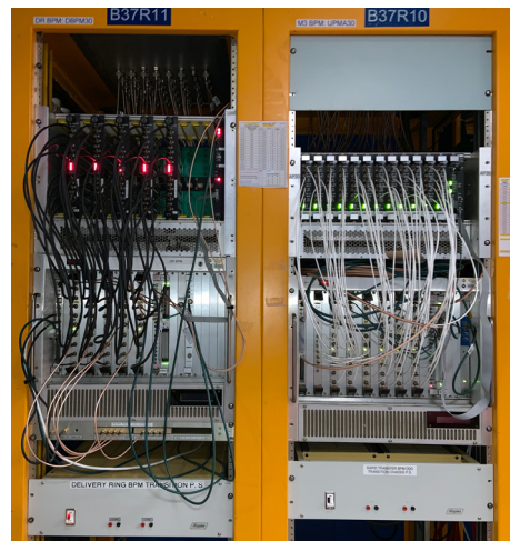
Figure 11: Layout of electronics rack (Delivery Ring: left, Transfer Line: right).
