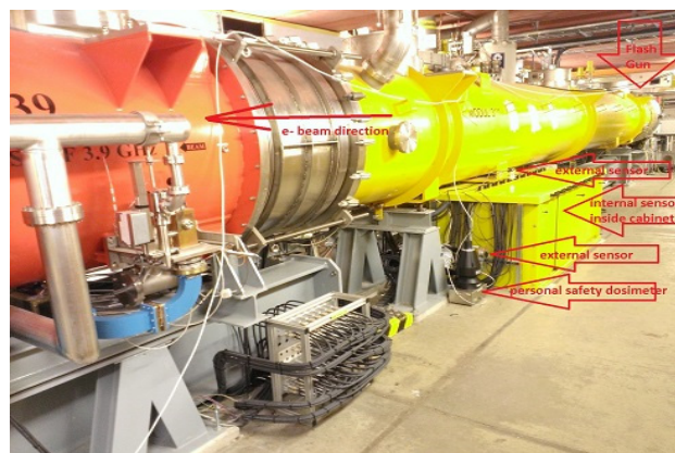
Figure 2: Flash RF-gun rack DosiMon system setup [5].
