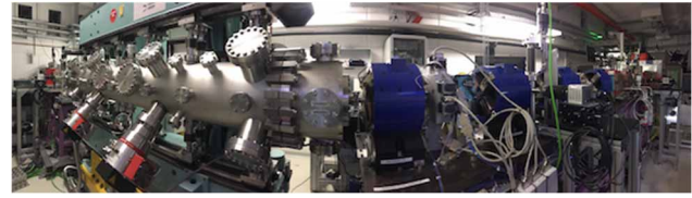
Figure 1: COXINEL line installed in HZDR LPA cave
