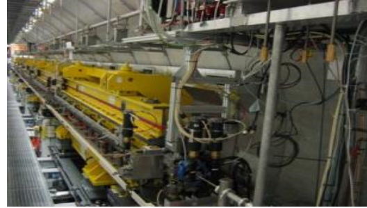
FLASH1 fixed gap undulators
