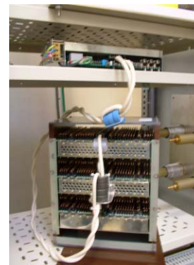
Figure 3: HV switch with its driver box (up).
