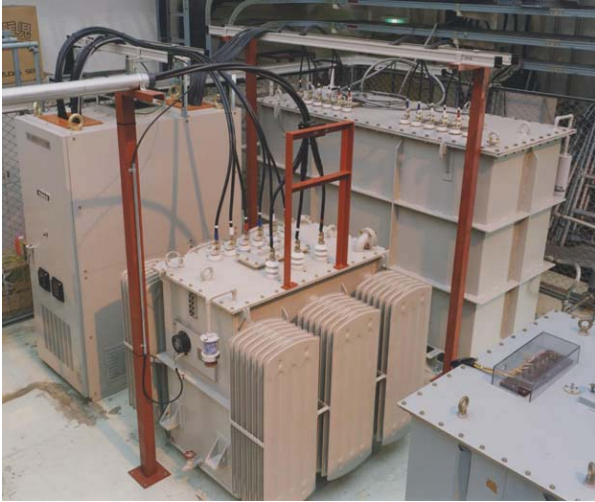
Figure 2: New klystron power supply as installed.
