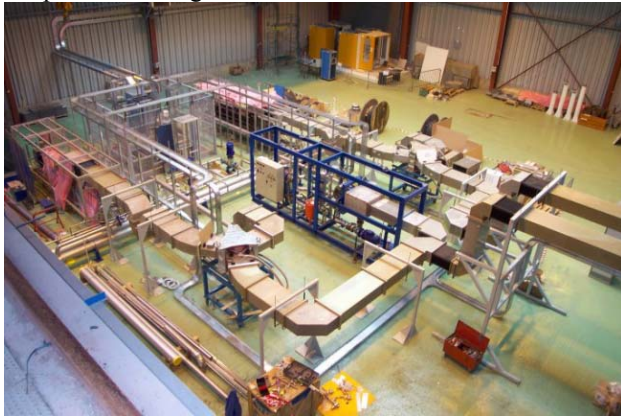
Figure 5 : View of the RF power system assembly.
