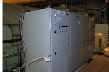
Figure 8: Power supply of kicker magnet
