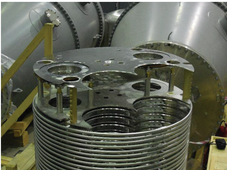
High voltage column
