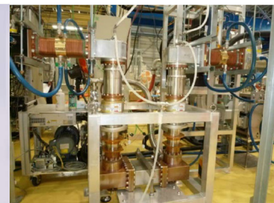
High power test stand
