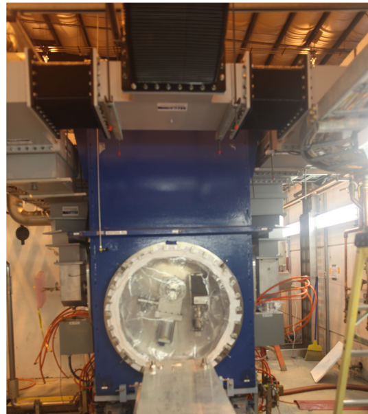
Figure 5: The SRF Photocathode electron gun installed in the ERL vault, as seen from the cathode insertion side. Notice the dual waveguide system of the fundamental power couplers.
