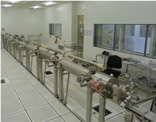
Figure 4: PXFEL2_2 in the ISO4 clean room facility
