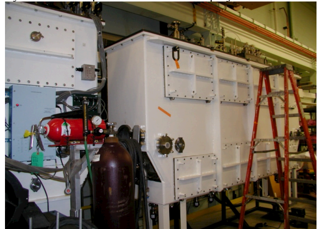
Figure 3: First two cryomodules installed and under testing in the ReA3 linac.
