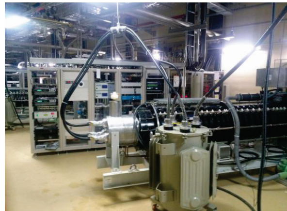
Figure 5: Control racks including LLRF system.
