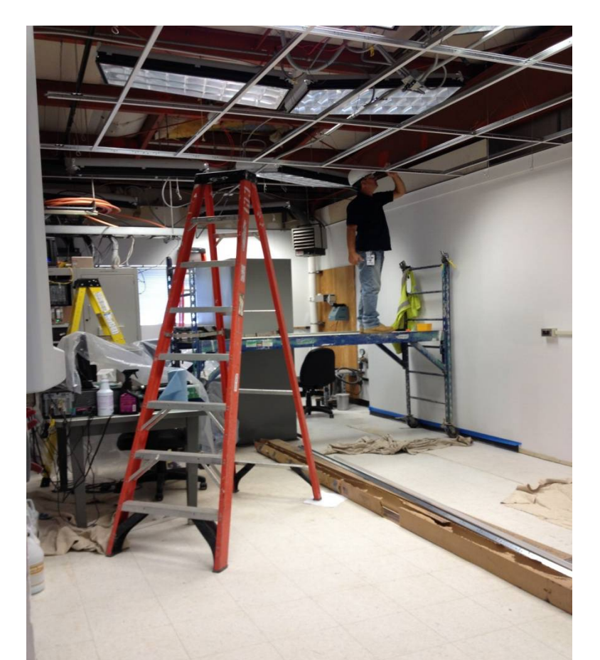
Work underway in BLIP control room where new electronics will reside
