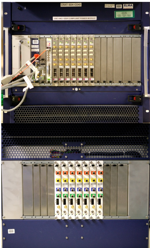
Figure 11: Seven BPM systems operating in a 12 slots ELMA crate.
