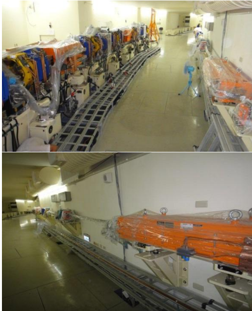
Figure 8: TPS installation. The left arc of upper figure is storage ring; the right arc is booster synchrotron. The lower figure shows the booster magnets which are fastened on the wall.
