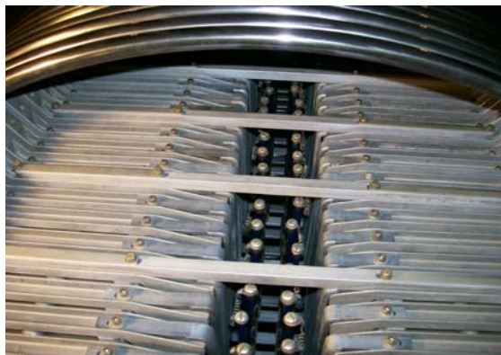
Figure 1: The new terminal voltage resistive divider installed between the column sections.
