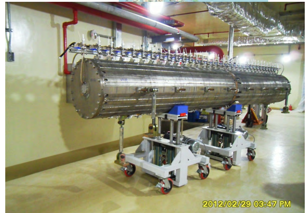
Special supporter inside tunnel
