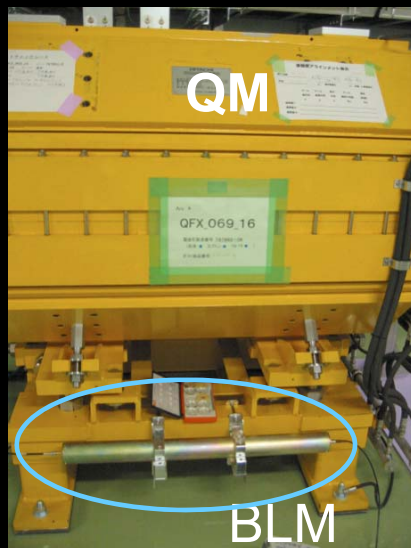
BLMs have been installed at each QM
