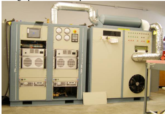
Figure 6: The 187 MHz 120kW CW RF source unit.
