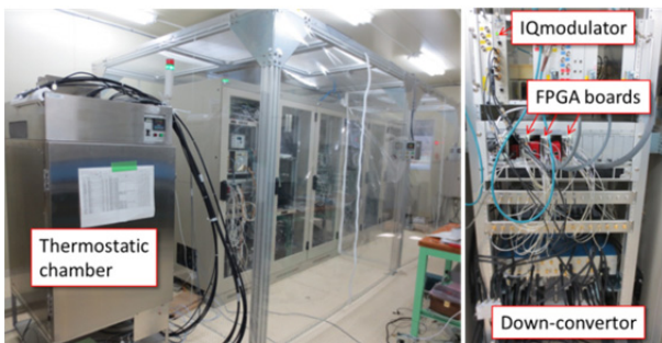
Figure 4: LLRF control racks.
